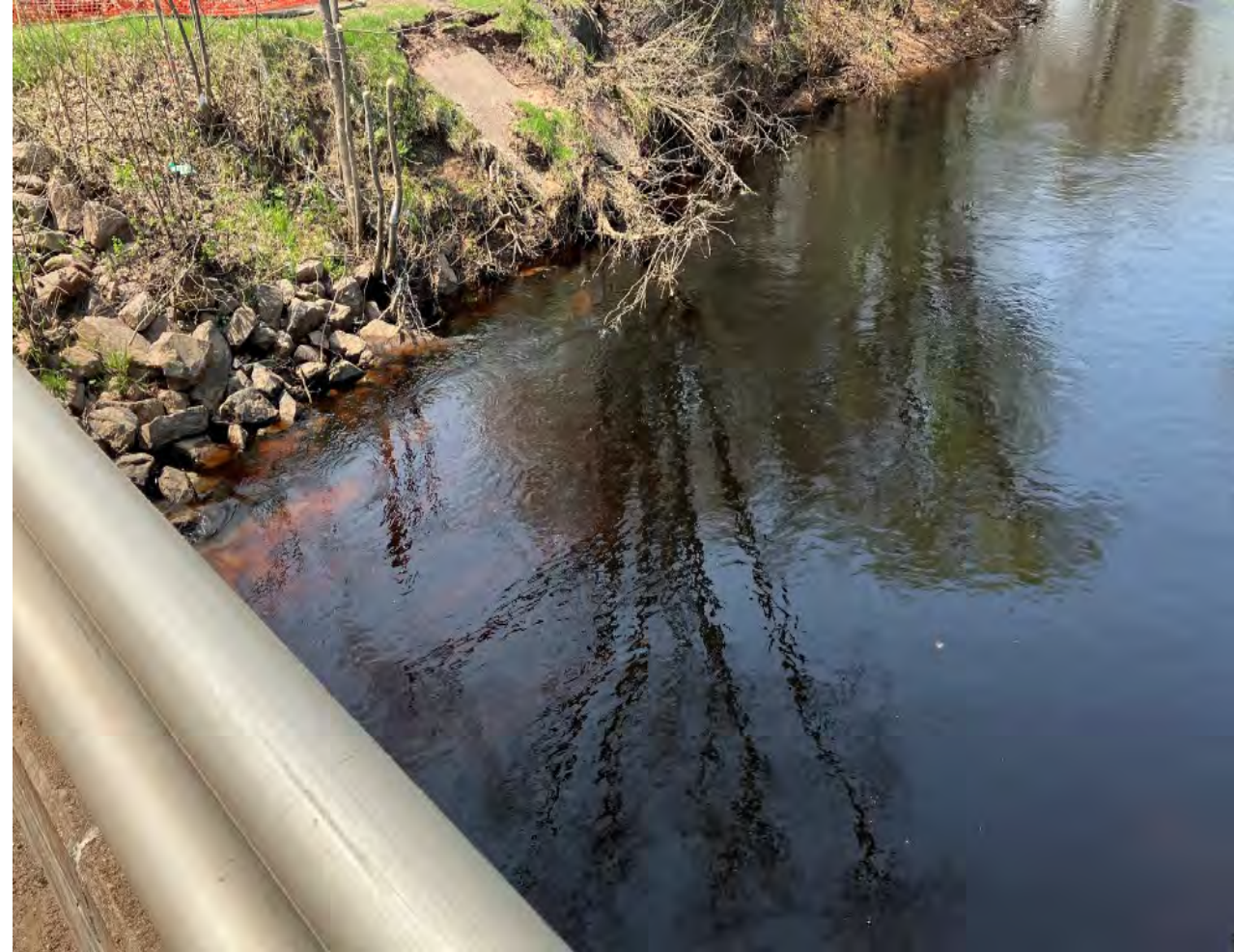
Bad River, Mellen, WI – site of Inadvertent Release incident during HDD, DOT project, 16 May 2023.
